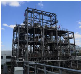
Fig. 2 Dual Fluidized Bed Gasification Pilot Unit
